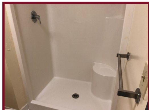
Bathroom - Shower Stall
